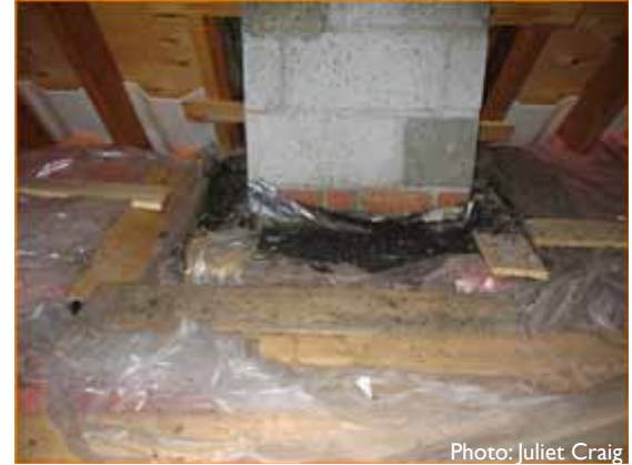
MODIFICATIONS FOR BAT ROOST SITES: PLASTIC SHEETING IN ATTIC TO FACILITATE GUANO REMOVAL AND REDUCE SMELL.
