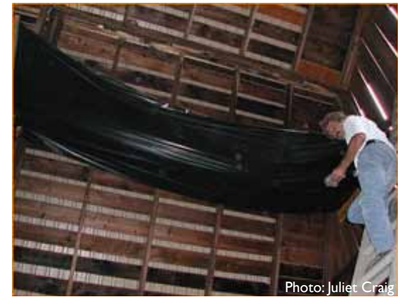
MODIFICATIONS FOR BAT ROOST SITES: TARP HUNG TO PREVENT GUANO FROM FALLING ON HAY.
